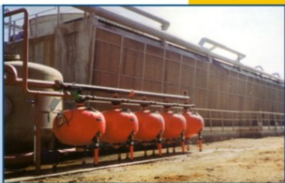
Cooling Tower Sidestream 150 m 3 /h 660 G.P.M
