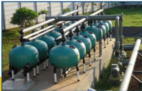
Drinking Water - Indonesia 200 m 3 /h 880 G.P.M
