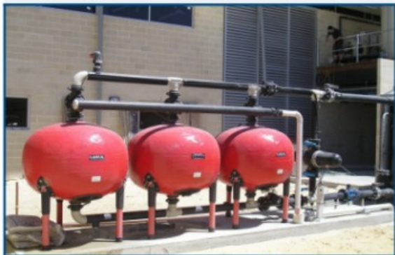
Seawater Aquarium 75 m 3 /h 330 G.P.M
